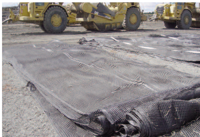
Due to the flexibility and ease of handling of the Miragrid® 8XT, the contractor was able to precut to embedment lengths prior to placement.
