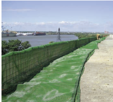
Facing installation showing Miramesh® GR draped over the wire mesh used as form work.
